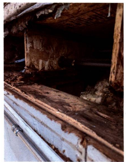
JOIST BEARING DAMAGE AT SAUNA
