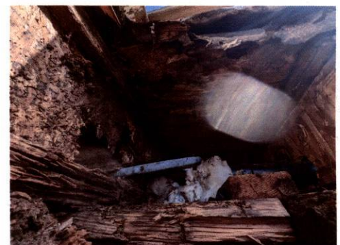
DECK, WEB, AND PLATE DAMAGE AT SAUNA
